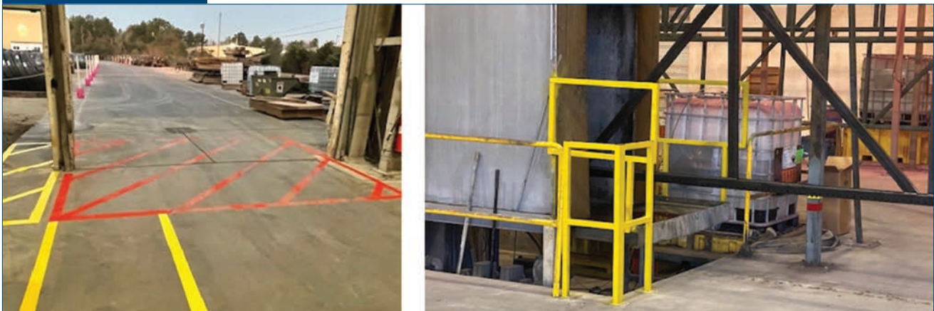
Safety upgrades at Nucor Warehouse Systems, which included painting walkways and adding guard rails.
