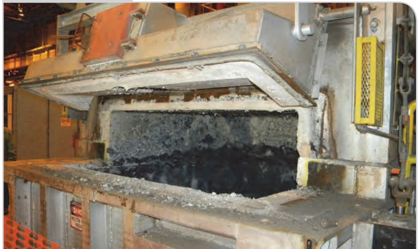
New footed door and view of cylinder and turnbuckle to the right.
