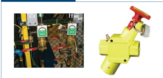
Maintaining a unique appearance and singular function of energy isolation devices in the mill may avoid potential confusion.
