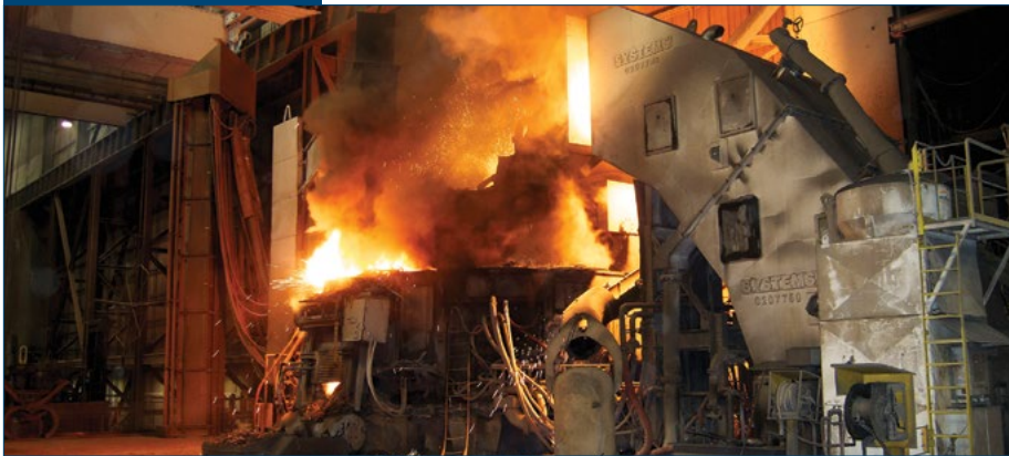
Spray-cooled furnace and duct.
