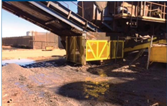
Potential hazards to individuals crossing under the conveyor.
