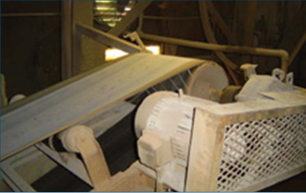
A typical belt conveyor installation.
