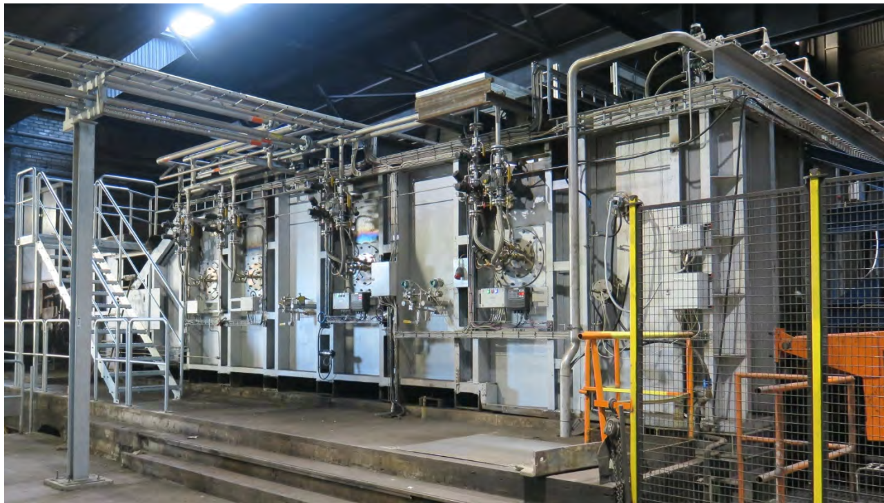
Figure 8. A reheat furnace at Ovako Boxholm, equipped with a hydrogen-ready REBOX Flameless Oxyfuel system. Installation and commissioning took place in 2024.
