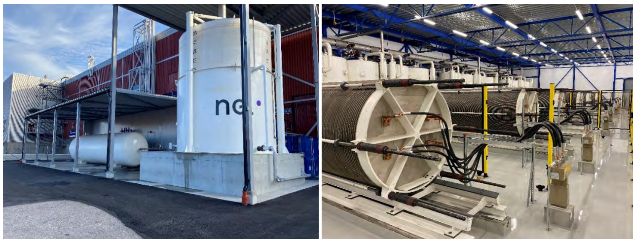
Figure 7. The 20 MW alkaline electrolyzer plant, which provides hydrogen to the operations at Ovako Hofors.
