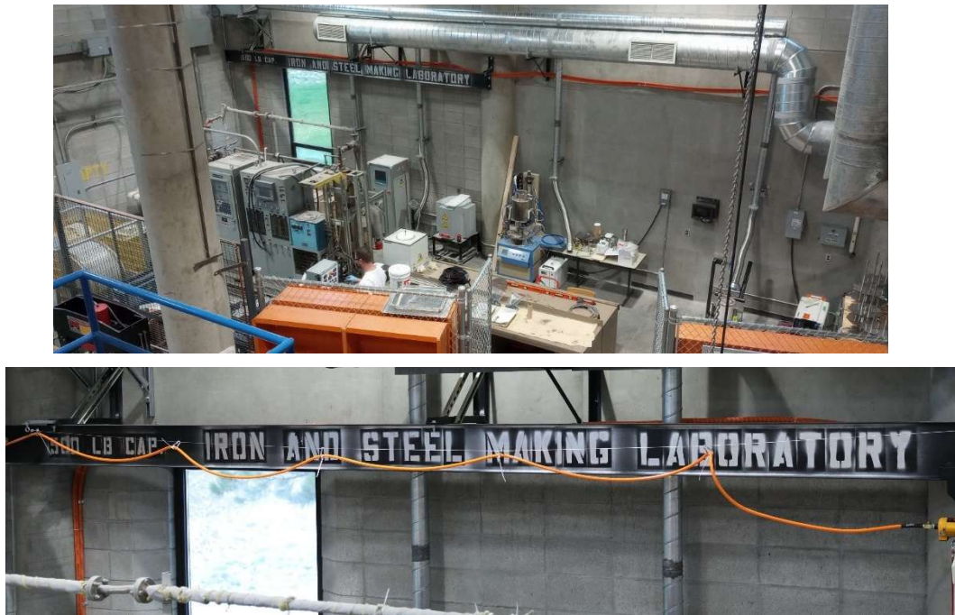
Figure 13. Pictures of the I&S Laboratory.
