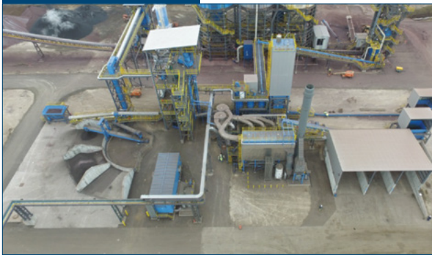
A cold briquetting plant for byproducts as an integrated part of a DRI plant at voestalpine Texas LLC.
