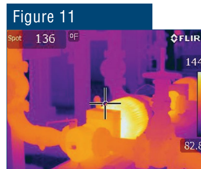
A lead and lag pump set. Both pumps are running but only one is moving fluid.
