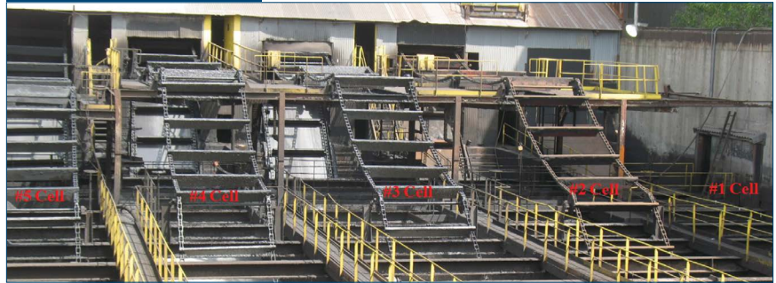
The #2 scale pit of a hot strip mill.
